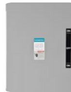
Manual Transfer Switch Subpanel
